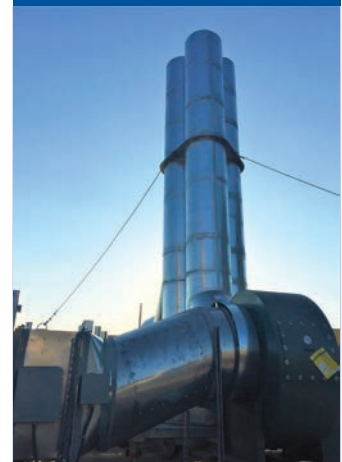
FIGURE 14 Close-up of cluster stack from performance design option installed
