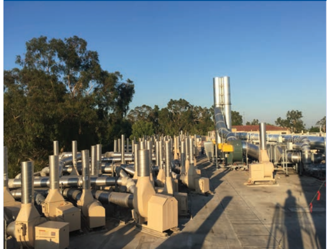
FIGURE 13 Performance exhaust stack design installed.
