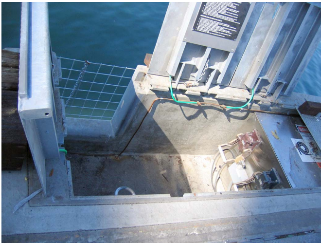
Fig. 1 6.6 kV connection box on wharf
