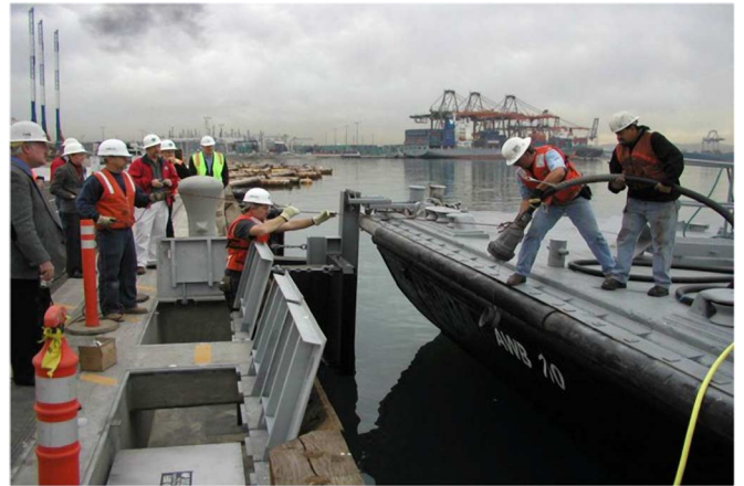
Fig. 1. 6.6-kV connection to shoreside power at POLA.
